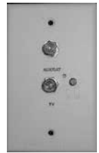
Antenna Power Supply
