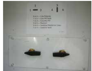
Fig. A -Water Valve Controls
