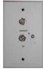
Antenna Power Supply
