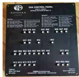
GFCI Breaker Panel
