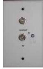
Antenna Power Supply
