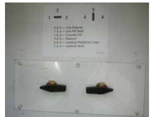
Fig. A -Water Valve Controls
