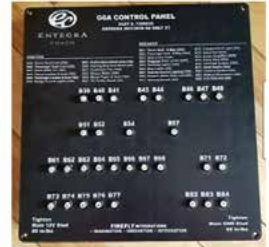
GFCI Breaker Panel
