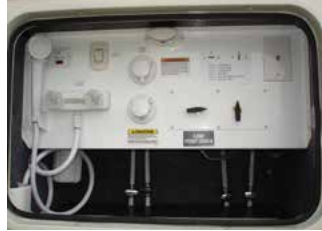
Fig. B - Utility Center
