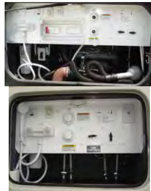
Fig. B - Utility Center
