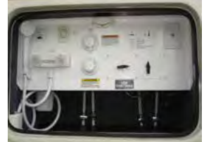
Fig. B - Utility Center
