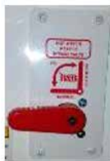
Water Heater Bypass Valve
